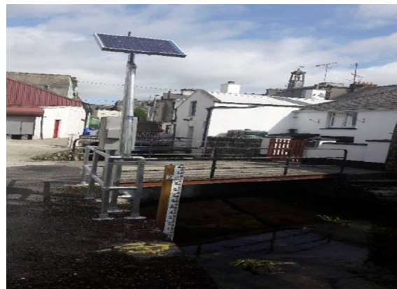
New Water Level Gauge – Turf Market
