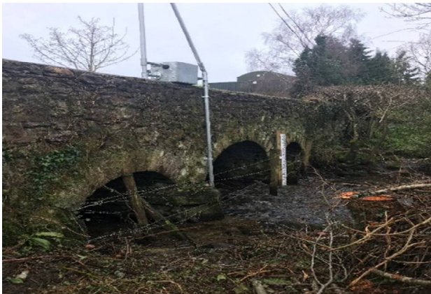
New Water Level Gauge – Coolroe
