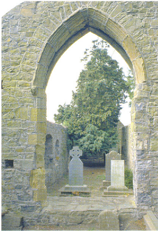
Above The use of cement mortar and ribbon pointing, as shown here, is inappropriate in the conservation of medieval buildings.
